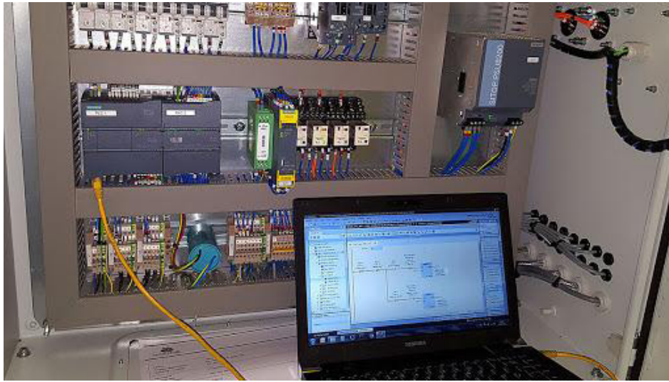
Figure 3: Programming the PLC
